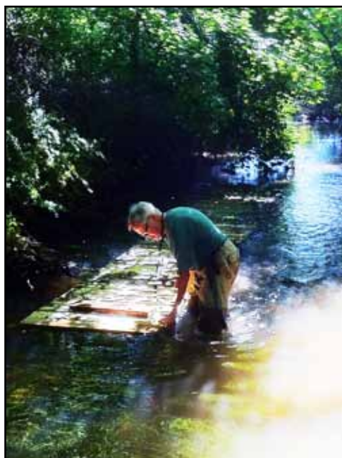
Volunteer Steve Gruber wades into knee-high flood waters to repair damage done to GSWA's Conservation Management Area by Hurricane Irene, August 2011. The storm caused severe flooding throughout the watershed for several days. Photo courtesy of John Neale.
