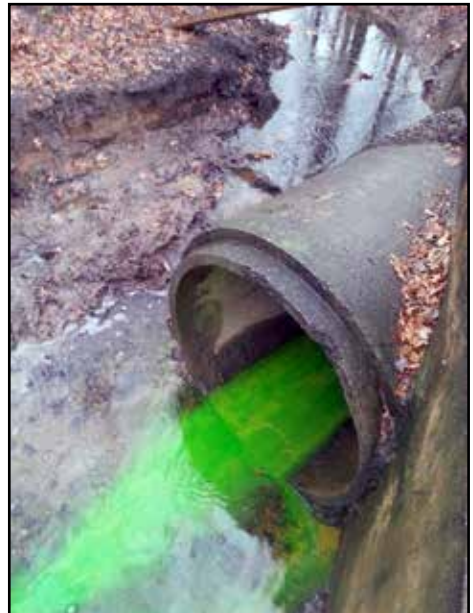
Biodegradable dye was used to trace the pipe to a storm drain in a nearby development. Credit: A. Follett.
