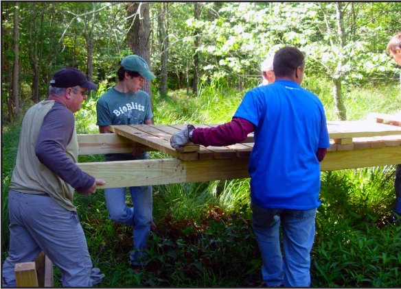
Volunteers construct part of a wooden boardwalk for installation at GSWA's Conservation Management Area in Harding Township, NJ. 2012. Credit: GSWA/H. England
