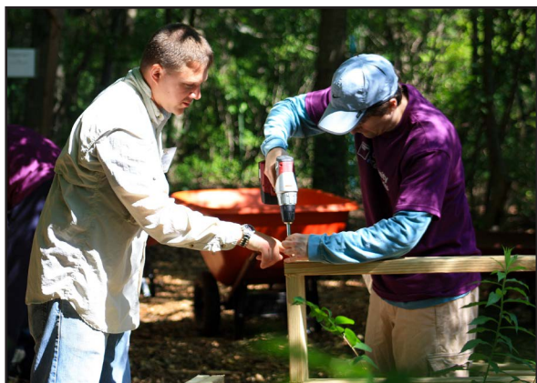
Volunteers construct part of a wooden boardwalk for installation at GSWA's Conservation Management Area in Harding Township, NJ. 2012. Credit: GSWA/H. England.
