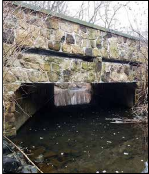
Beautiful bridge as the Passaic River runs under Tempe Wick Road in Mendham, near the headwaters of the river.
